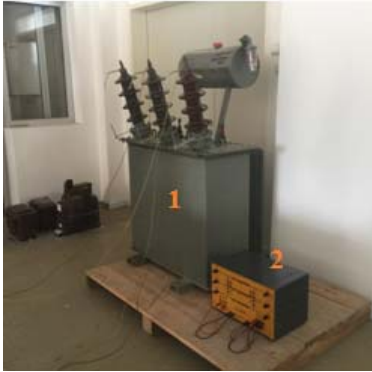
Fig. 4. 50kVA, delta/star, 34.5/0.4kV distribution transformer for PLC. (1) distribution transformer, (2) line model
